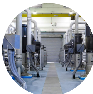
Minimal Liquid Discharge
