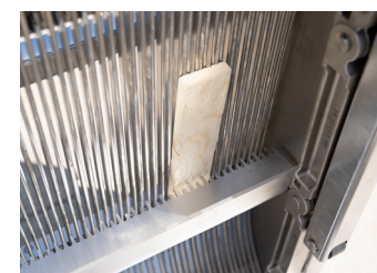
C Rapid re-engagement removes large debris without shutdown to return scraper into the bar screen faster
