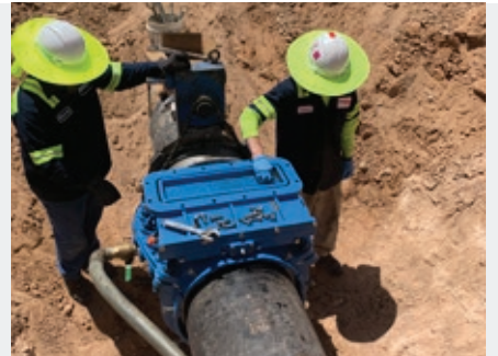
5 | Integral Isolation Gate is closed to prevent water loss
